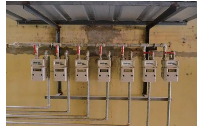
Meter installation site
